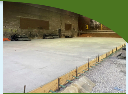
Carroll County Transfer Station Bays 1 & 2 concrete slab and drainage layer beneath slab (#57 stone)
