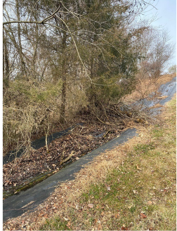
Vegetation obstruction of Cell 4 Hypalon Ditch #1 (5)
