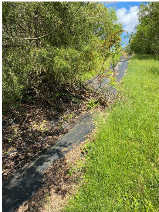
Hypalon Ditch #1 vegetation obstruction
