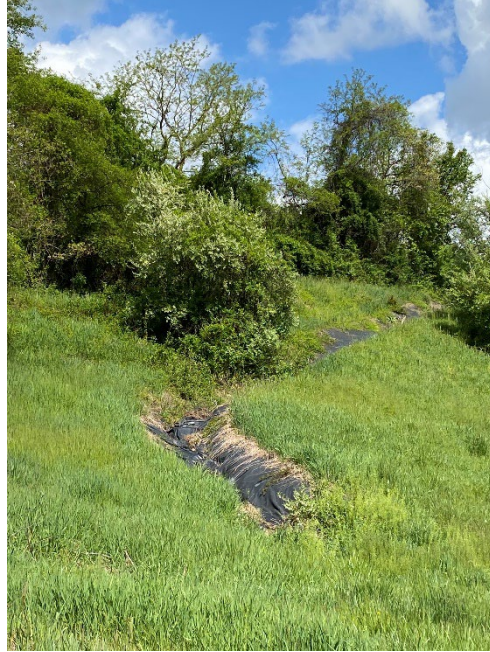
Hypalon Ditch #1 vegetation obstruction
