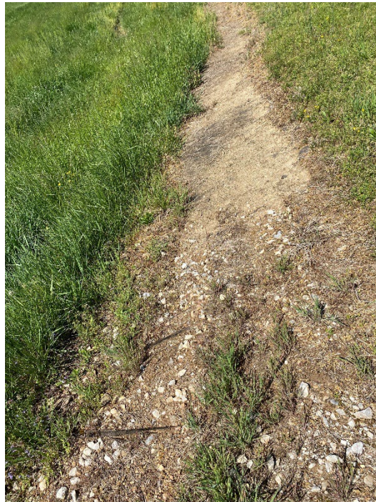
Erosion and exposed liner on Southeast slope
