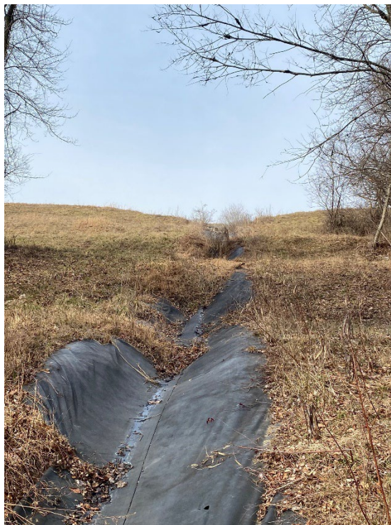
Settled dirt and growing vegetation on Cell 1 Hypalon Ditch #3 (3)
