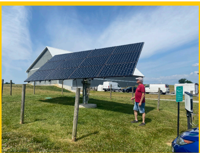
In addition to being a 100 percent solar powered winery, Linganore Winery parking areas have complimentary solar chargers.
