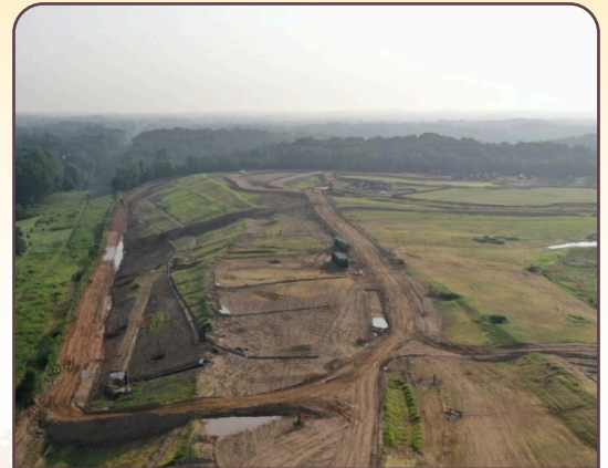
Access roads constructed in Phases S-I and S-II this summer will facilitate the placement of the subgrade layer installation.
