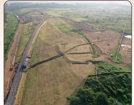
Wastes excavated and relocated in Phase S-III in July. Grass seed stabilized the soil post-excavation.
