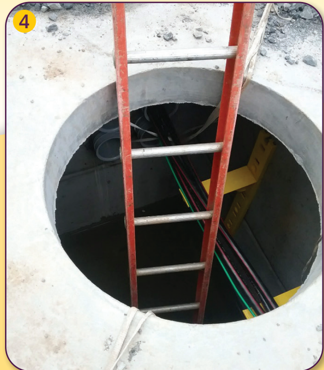
Manhole showing the cabling (medium voltage power and communications). (01.10.2020)
