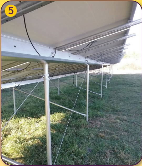
Under side of the panels, showing the connected wiring. (01.17.2020)
