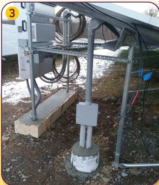
Side view of the solar array, showing the inverter, cabling, and mow strips in forms. (01.10.2020)
