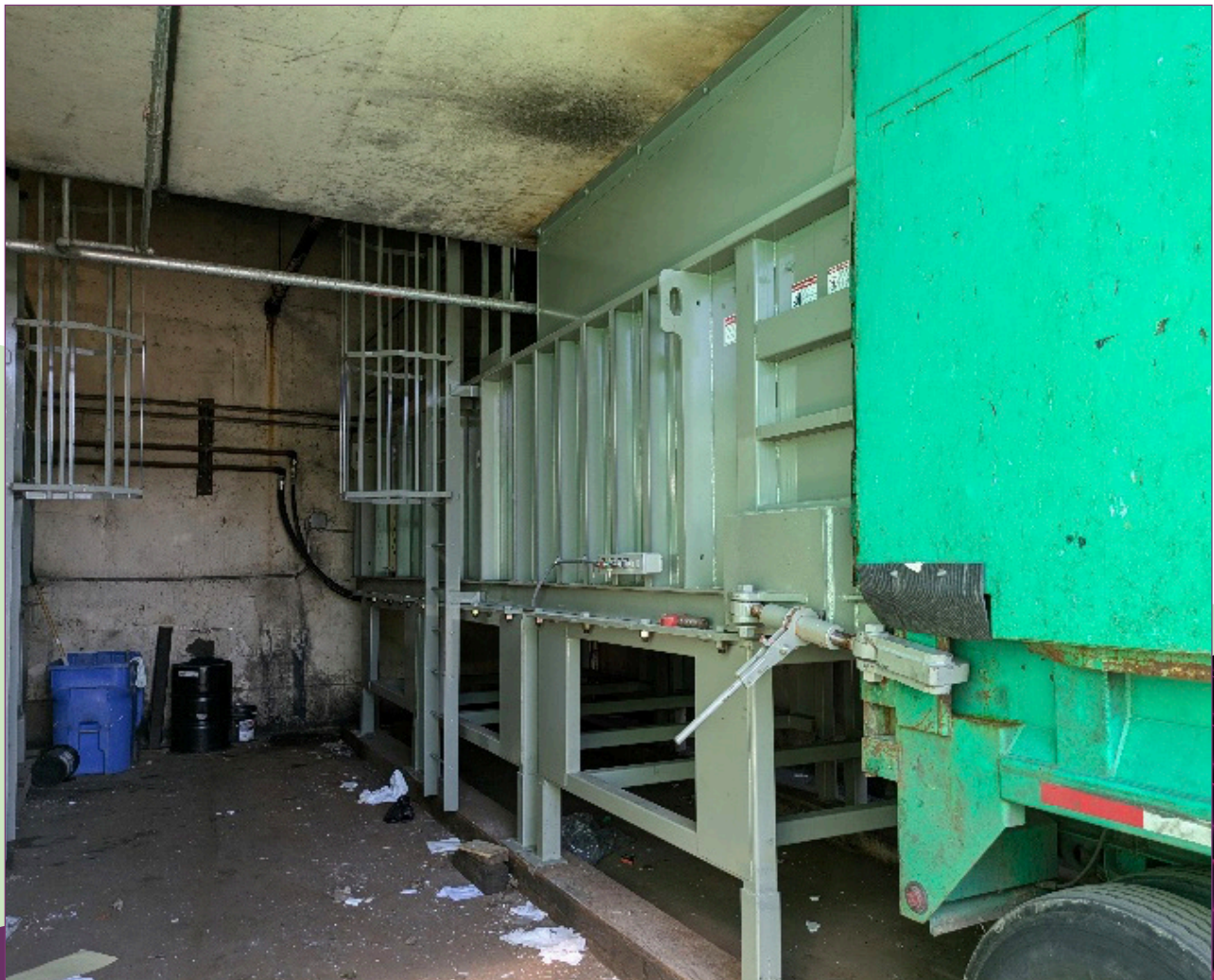
A tractor trailer maneuvers a new transfer compactor into place at the Northwest Transfer Station.
