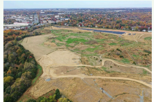
Phase III after geosynthetic liner placement and Phase V before disturbance from October 2023
