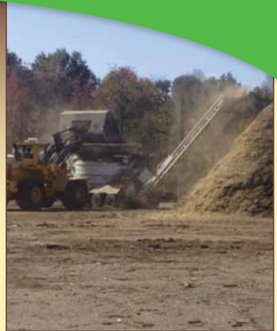
Materials received at the Western Branch Composting Facility are ground in a horizontal grinder prior to being placed in windrows.
