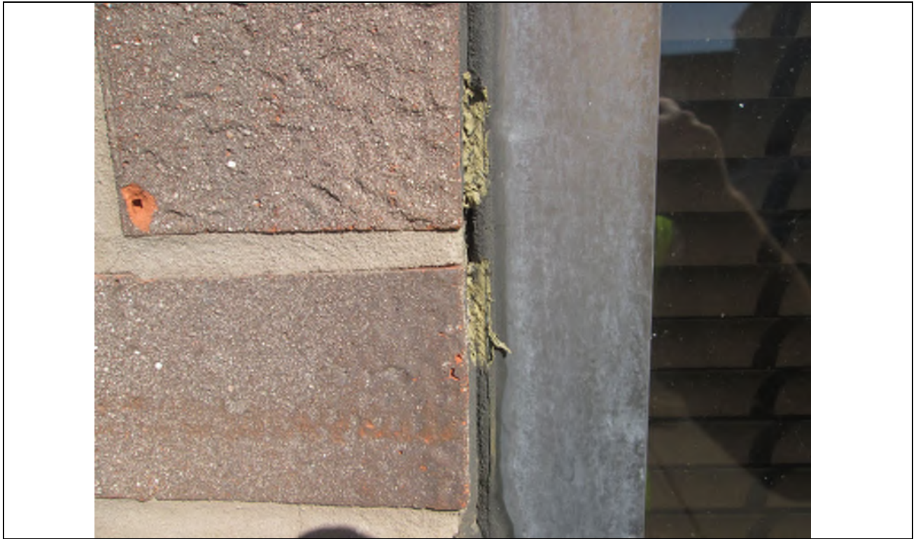
Photo No. 3: View of interior/exterior window casing caulk of the Office area which was determined to contain 6% to 8% Chrysotile via PLM analysis of bulk samples.
