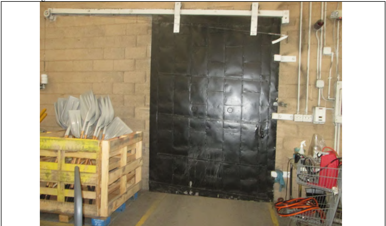
Photo No. 8: View of metal sliding door between Warehouse (black side) and Garage (white side) determined to be coated with LBP via XRF testing.
