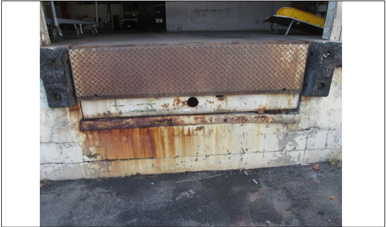
Photo No. 13: View of white metal plate on face of lift gate at loading dock exterior determined to be coated with LBP via XRF testing.
