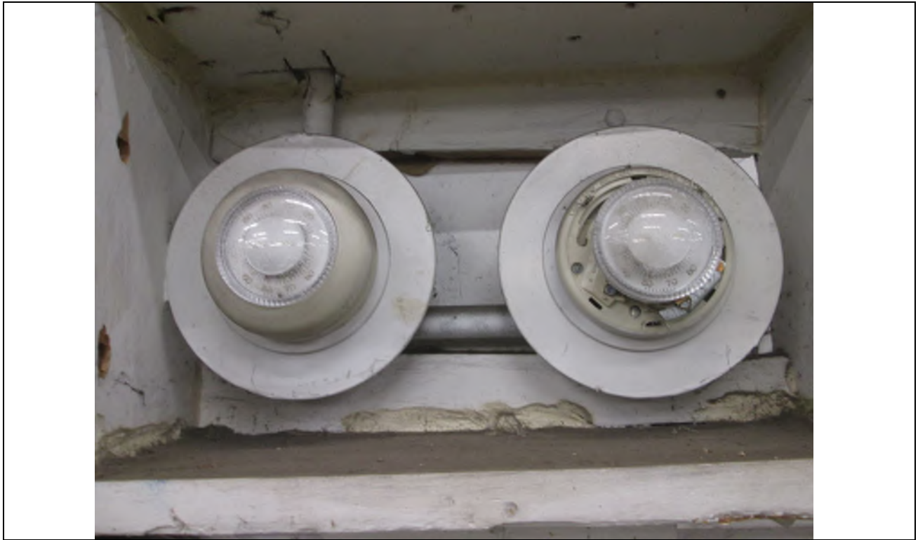
Photo No. 21: View of thermostats observed in the Warehouse area (Side C) with mercury bulbs.
