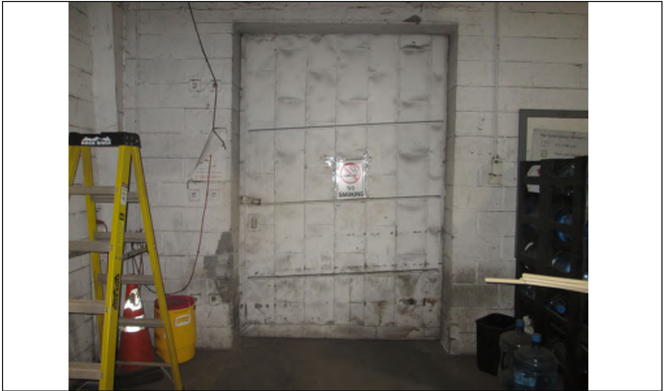
Photo No. 7: View of metal sliding door between the Garage and Warehouse presumed to be asbestos containing.
