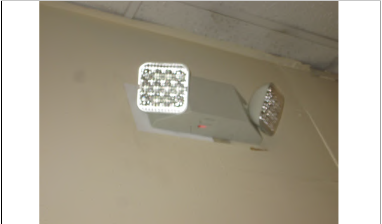
Photo No. 17: View of typical emergency light fixture observed in the building with one suspect battery and two suspect mercury-containing bulbs.
