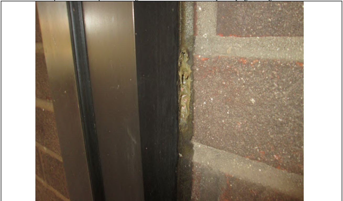
Photo No. 2: View of interior/exterior black storefront casing caulk associated with the glass/metal Foyer to the Office area which was determined to contain 8% to 10% Chrysotile via PLM analysis of bulk samples.
