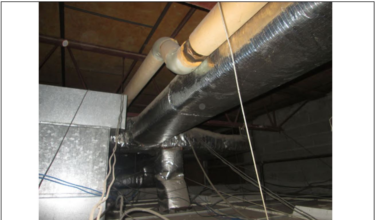
Photo No. 20: View of uninsulated duct, flex duct, fiberglass insulated duct, and fiberglass insulated piping observed above the ceiling in the Office area. No mastics/seam sealants were observed on these building components during the survey.
