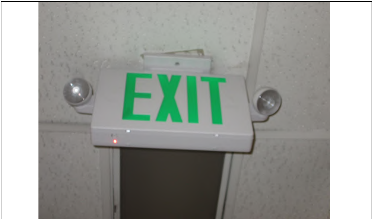
Photo No. 16: View of typical emergency EXIT sign observed in the building with suspect battery and two suspect mercury-containing bulbs.
