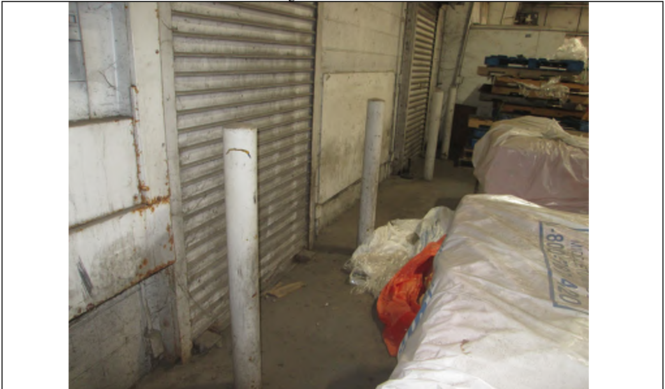
Photo No. 12: View of white metal traffic bollards in Garage and Warehouse determined to be coated with LBP via XRF testing.
