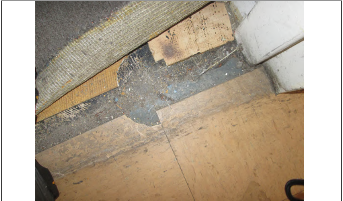
Photo No. 1: View of 12x12 tan VFT (below carpet) and associated black mastic found in Office area electrical closet which was determined to contain 3% to 6% Chrysotile. This tan VFT and/or associated residual black mastic is presumed to be present throughout the Office concealed by overlying flooring materials.
