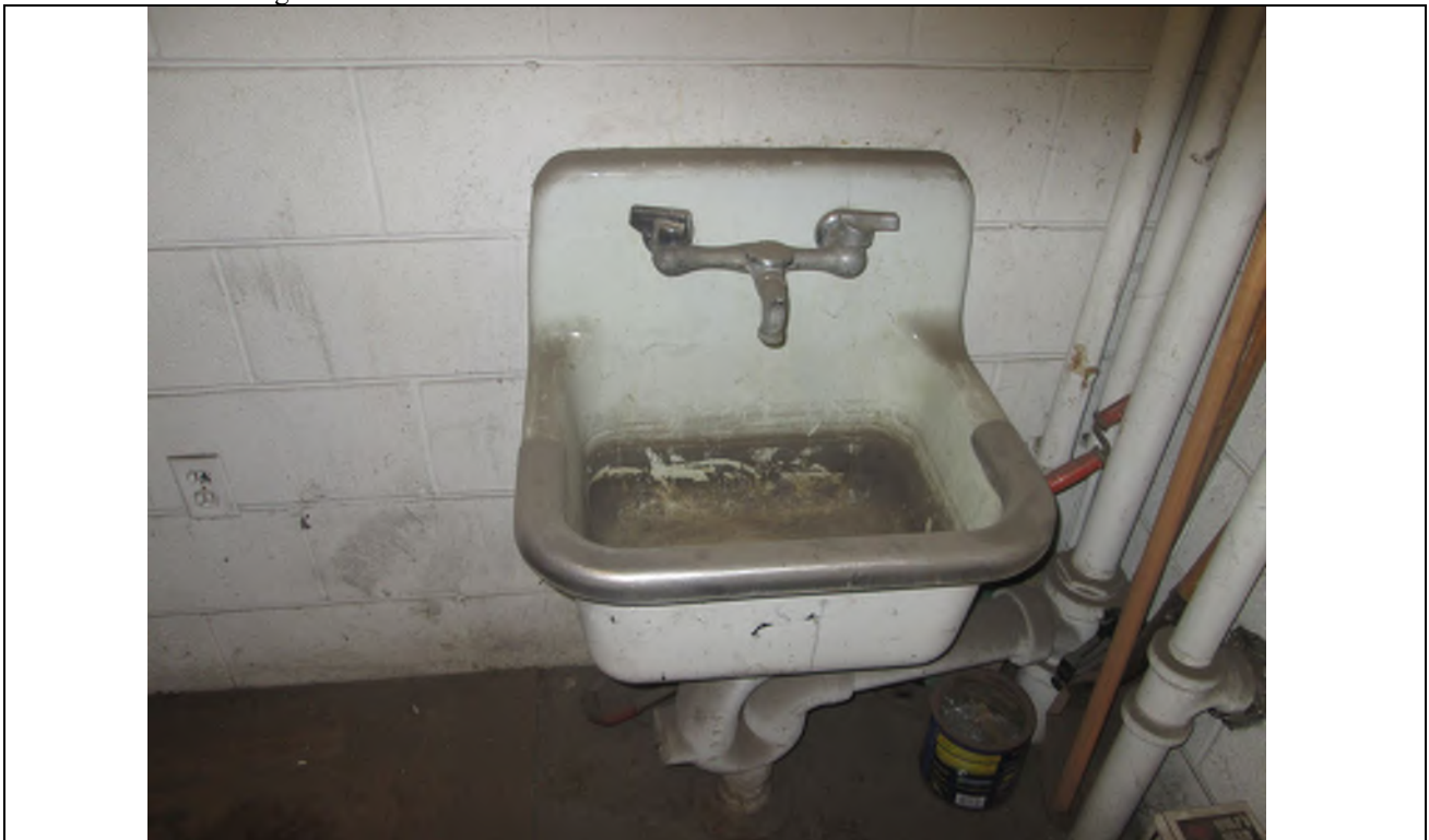
Photo No. 10: View of white metal slop sink in the Garage Janitor's Close determined to be lead based via XRF testing.
