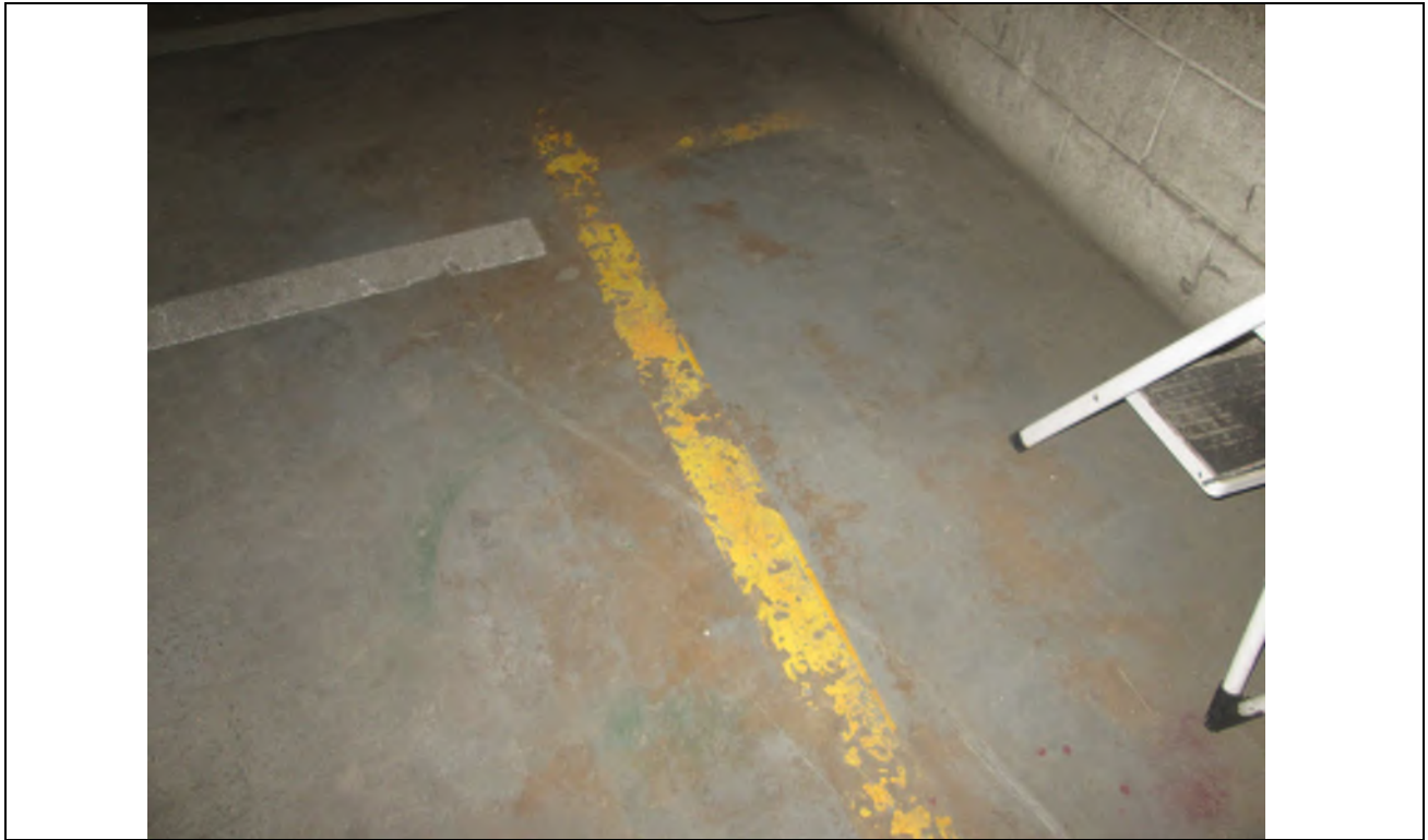
Photo No. 9: View of yellow traffic markings on concrete floors in Garage and Warehouse determined to be LBP via XRF testing.
