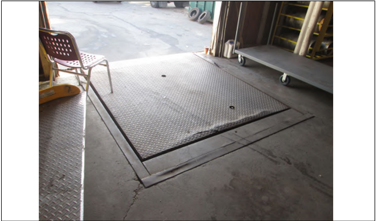
Photo No. 25: View of hydraulic loading dock lift gate with suspect oil reservoir observed in the Loading Dock area of the Garage.
