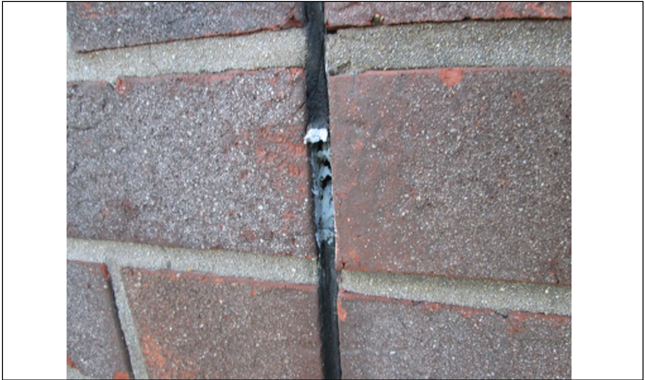
Photo No. 5: View of white exterior building caulk in vertical brick wall seams on the exterior Warehouse area which was determined to contain 10% to 12% Chrysotile via PLM analysis of bulk samples.
