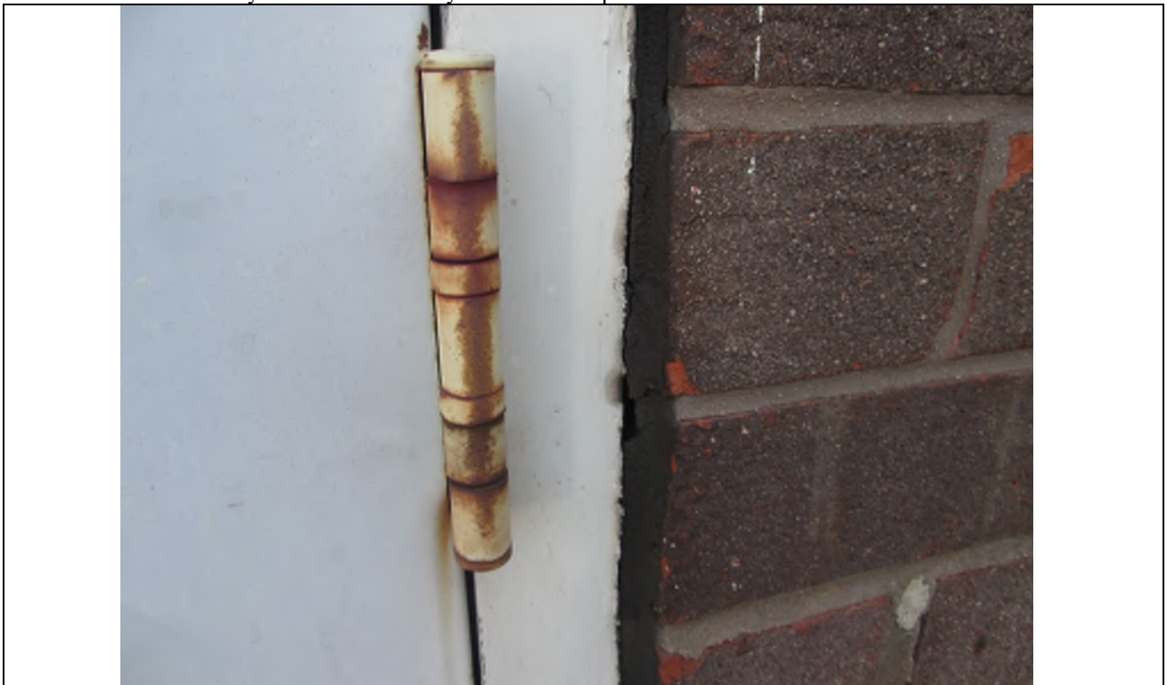
Photo No. 4: View of black exterior door casing caulk on Sides A and D of the Office area was determined to contain 6% to 8% Chrysotile via PLM analysis of bulk samples.
