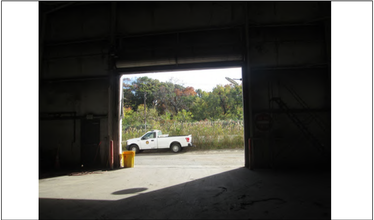
Photo No. 11: View of grey metal Garage Door Casing [center garage door only] along rear wall of Garage determined to be coated with LBP via XRF testing.
