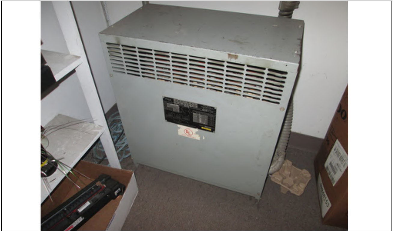
Photo No. 19: View of small transformer observed on the Office area electrical closet.
