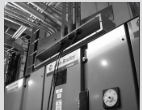
▲ The new Allen Bradley 4160 switchgear in the lime preparation building will service the power requirements of the new air pollution control equipment.
