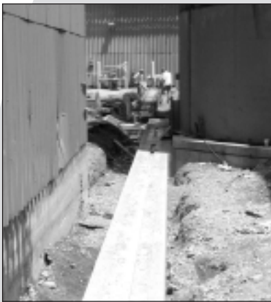
▲ A newly formed trench drain behind the lime preparation building will support the collection of stormwater.
