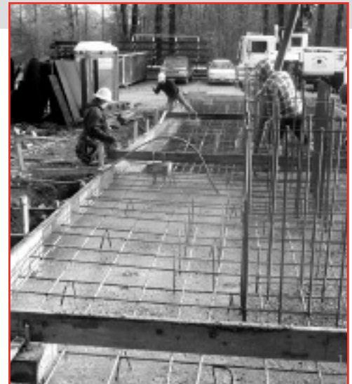
Foundations are being poured to support three new ID fans that will help pull the flue gas through the new emission control equipment.
