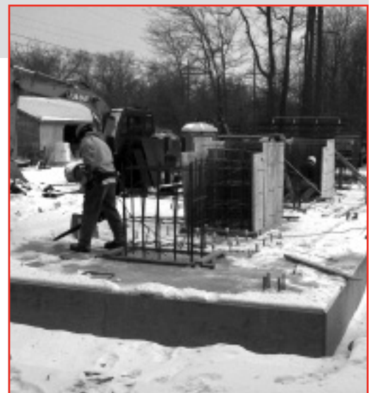
Work continues after the mid-January snowfall on forming the piers that will support the ID fans.
