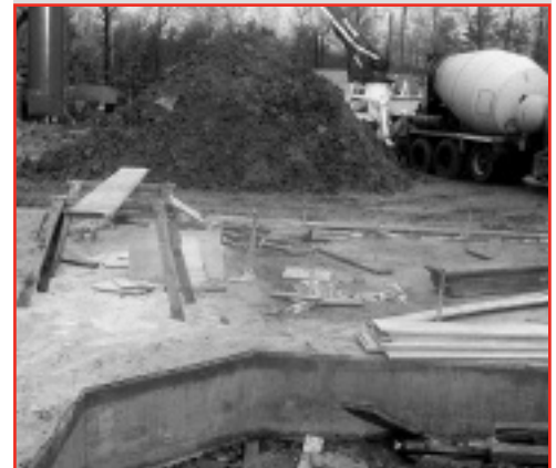
Completed foundation for the lime silo and lime slurry preparation equipment. The lime slurry will be injected into the acid gas scrubber to neutralize the acid gases in the flue gas.
