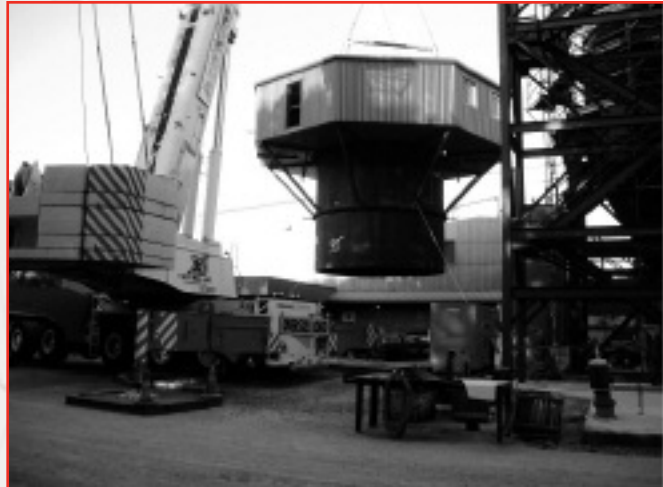
The top of the scrubber is lifted from the ground where it was fabricated.
