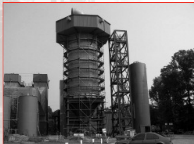
The inlet duct sits atop the scrubber. Adjacent to the stair platform is the lime preparation system.
