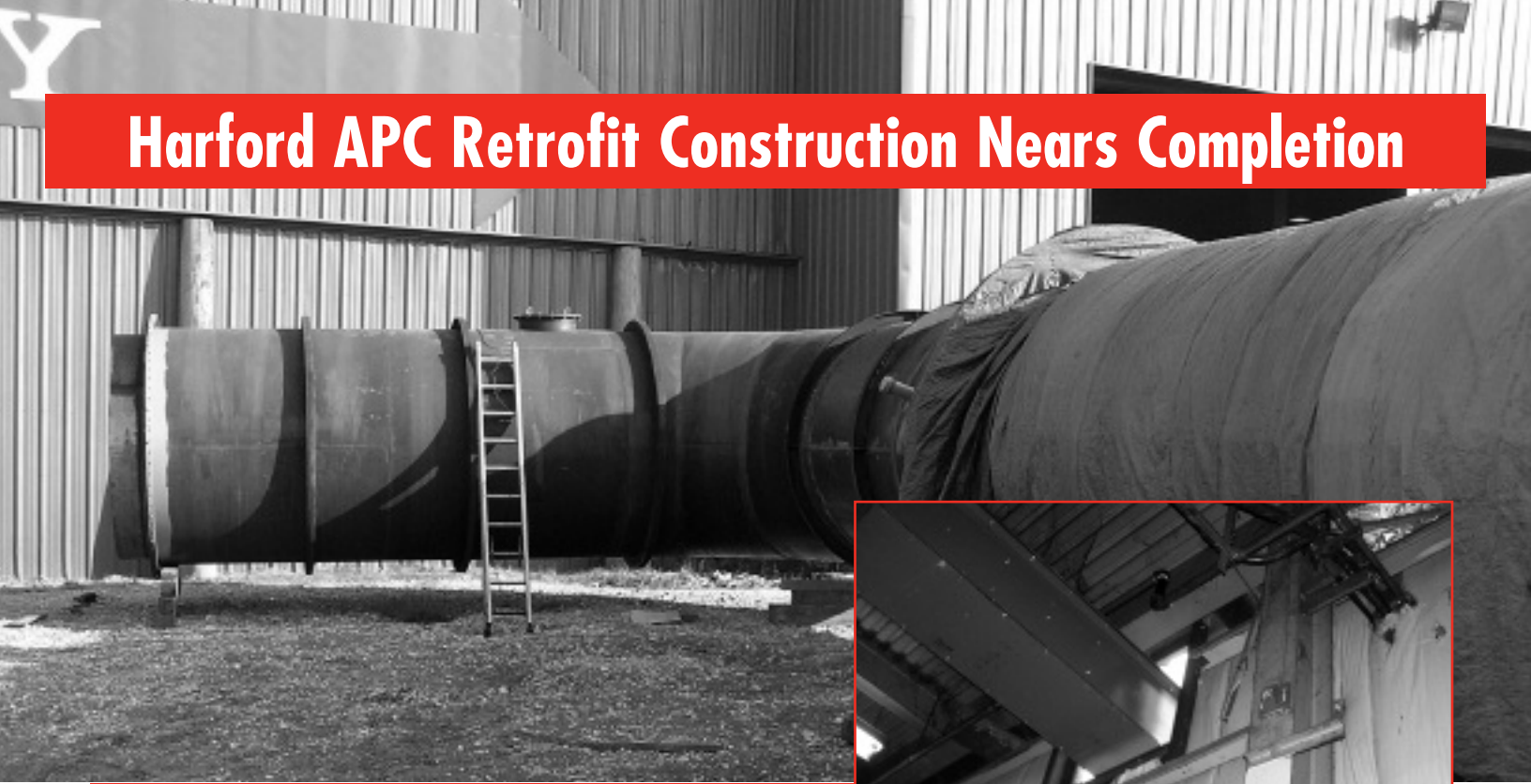
Above: large duct that will carry the flue gas to the top of the scrubber Right: ash conveyor as it enters the facility's vehicle maintenance shop
